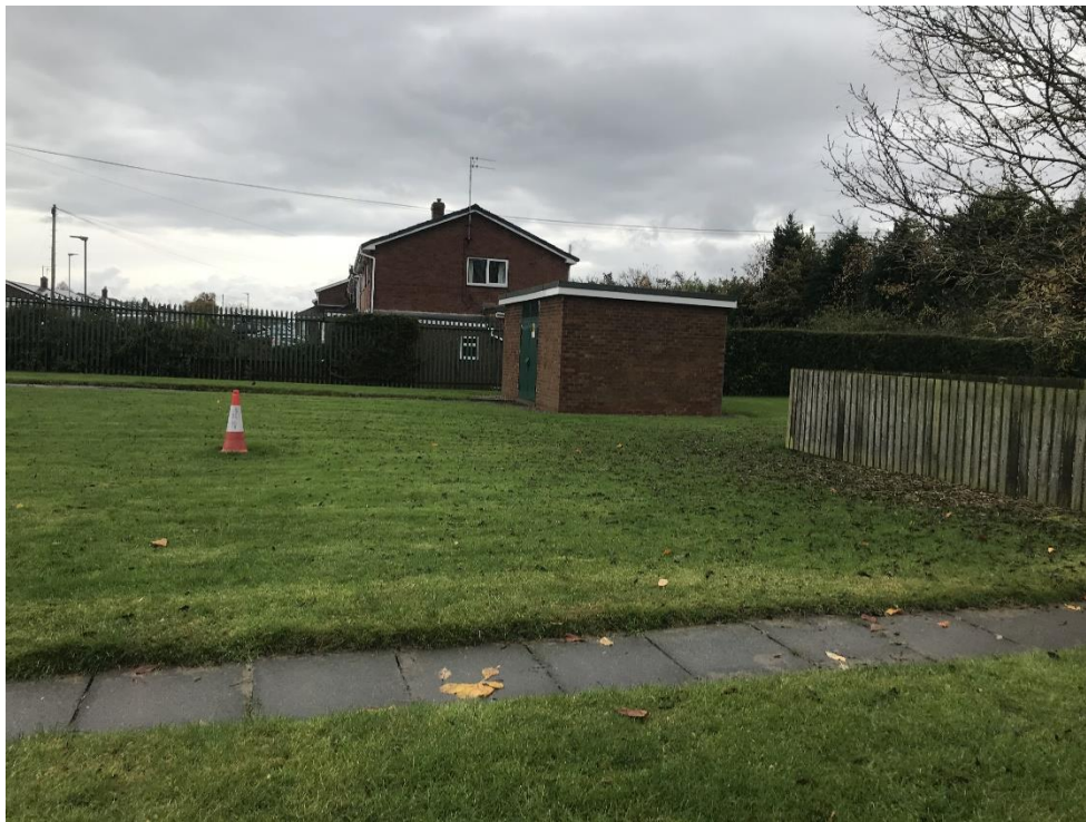
Photo 4: Showing the electrical substation present in the south eastern corner of the site.
